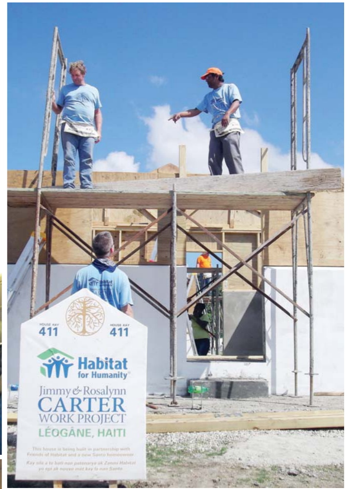
Each team was allocated two homes to complete. The houses were already built up from the foundation to about a metre and a half. It was our job to complete the rest of the house using timber. This included constructing the walls, putting in the roof trusses, knocking in the roof, installing the gutters, screwing in the sidings to make the walls look more appealing, hanging in the doors and windows and lastly, erecting a little porch at the house front. It was tough, but in the end rewarding work. Off course, in case you were wondering, not all the homes were completed. The plan was that a team of professional builders employed by Habitat for Humanity were to come in the following week and complete the homes, including partitioning the house into different rooms, installing the toilets, and connecting the water supply.
