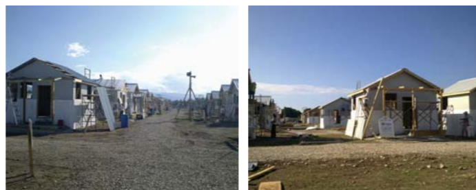
Our objective was to build 100 of these homes before the end of the week. (This photo is showing the houses almost at completion. When we got there there was only the foundation and the walls (white) constructed up to about a metre and a half. The enthusiasm and dedication that the volunteers displayed in trying to achieve this was a sight to behold – and this with no supervisor standing over your shoulder, and, sweltering heat and humidity to contend with.
